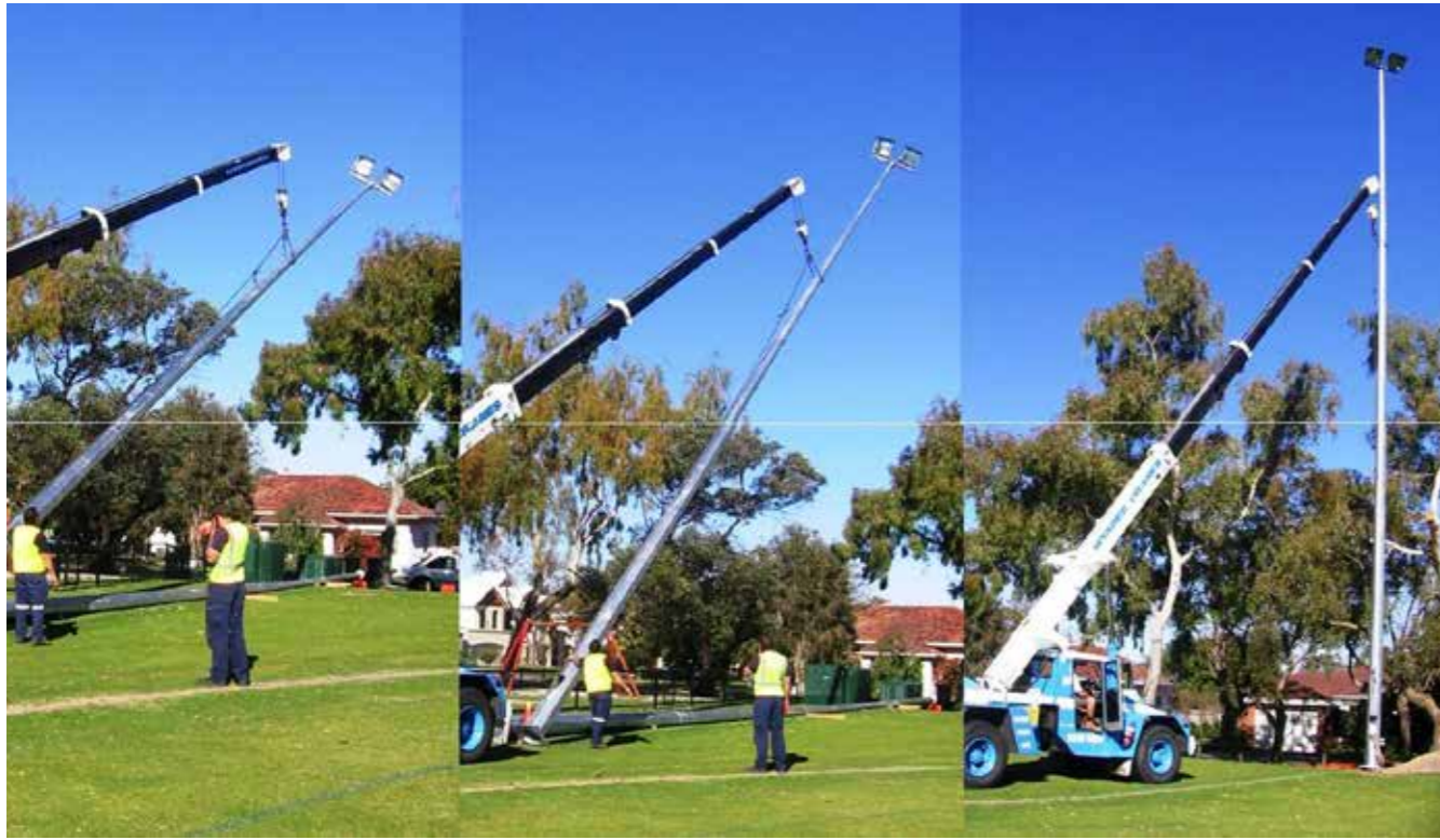
Erection of the two towers at the southern end of Gairloch Reserve occurred in August 2008. Provision for electrical connection to additional towers at the northern end was also installed. This was a positive step for better utilisation of the oval during training nights.
